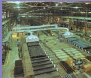
連続焼鈍炉 Continuous annealing furnace
