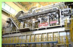
Energy-saving heating furnace that uses regenerative burners
