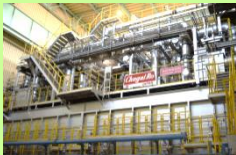
Energy-saving heating furnace that uses regenerative burners
