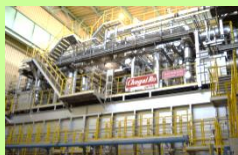
Energy-saving heating furnace that uses regenerative burners
