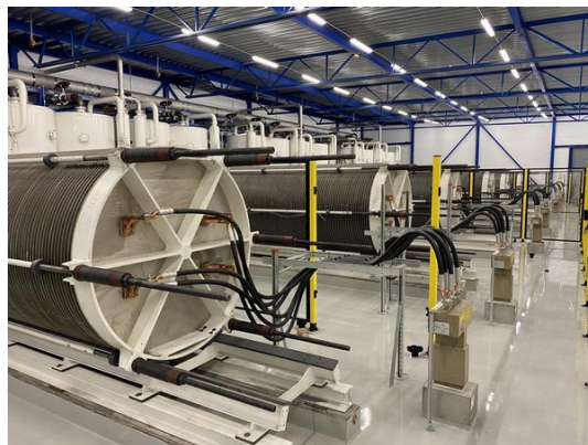
Electrolyzer of Hydrogen plant of Ovako
